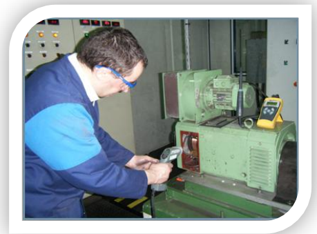
Control of the operating conditions
